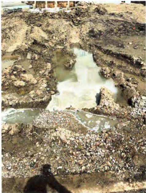
Concrete washout in tire tracks where the concrete trucks were entering the site via the ramp.
